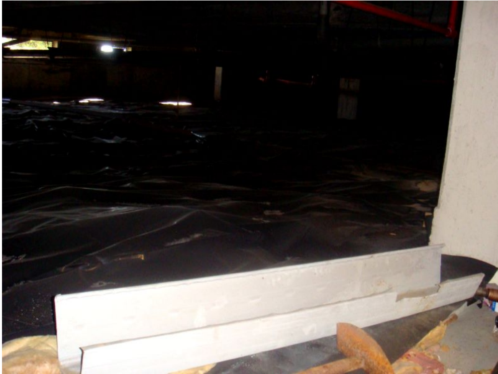
Picture – The black polythene on the basement floor is in place in order to encapsulate asbestos.
