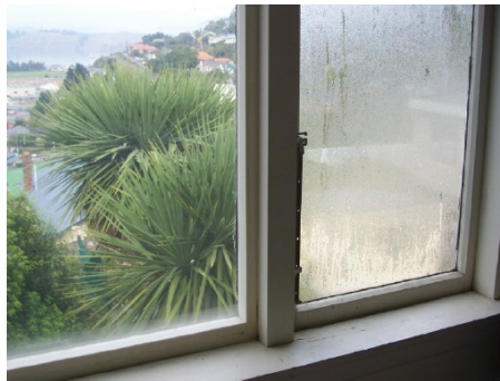
The left hand window is insulated using a window insulation kit. The right hand window is un-insulated, and continues to collect condensation and lose heat.
